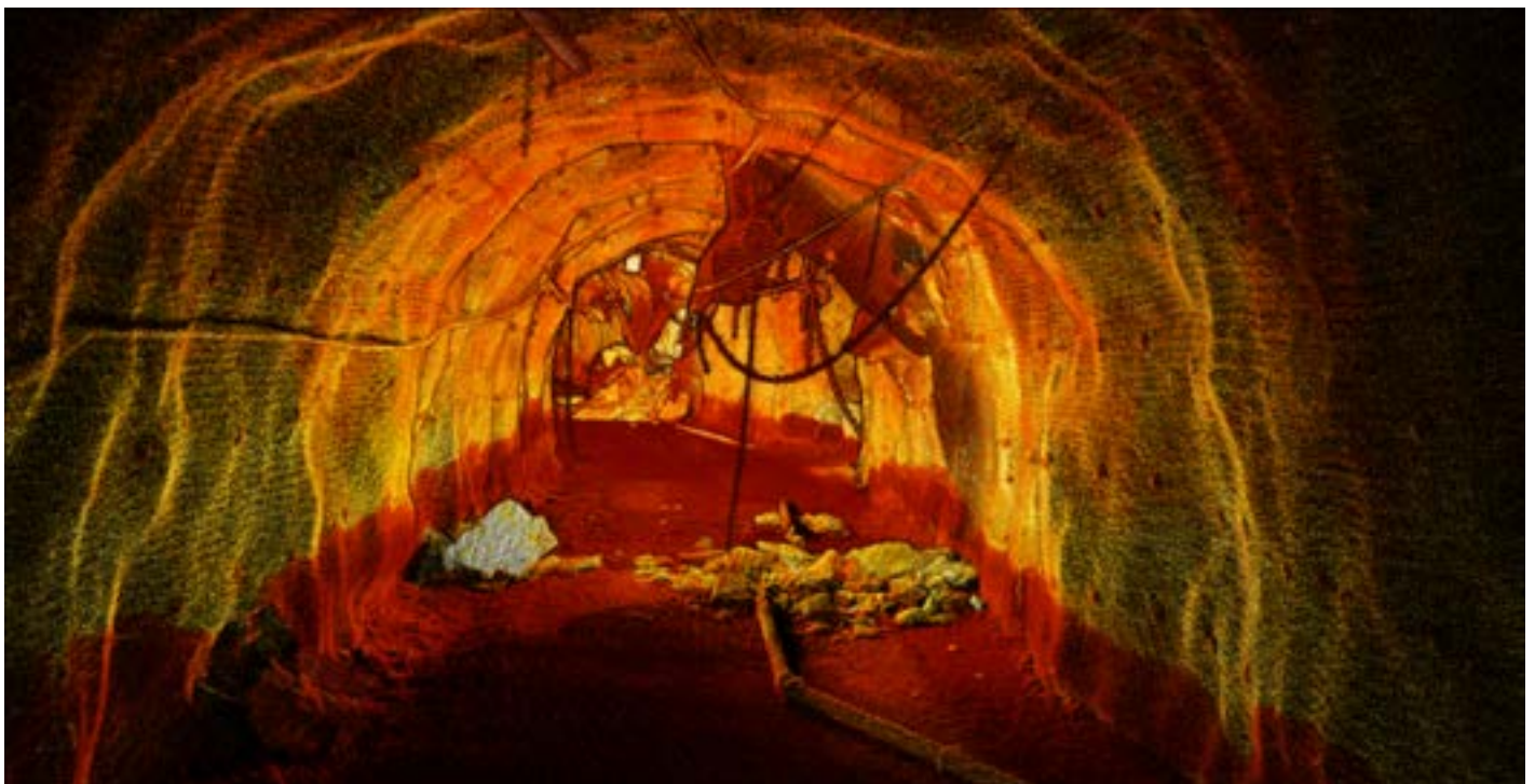
AMKVO delivered georeferenced point cloud data sets, still images and animated point cloud films. LKAB published the films to inform stakeholders, employees and local residents of the extent of the damage.
